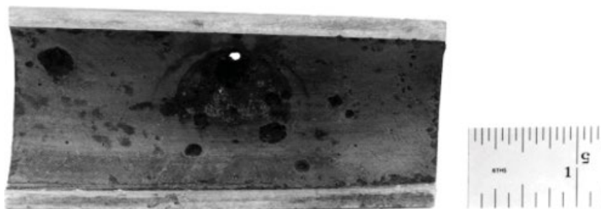
Figure 15—Boiler Tube Showing Penetration of the Tube Wall by a Localized Oxygen Pit
