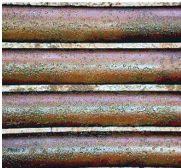
Figure 11—General Metal Loss and Pitting of Tubes Exposed to Moisture and Corrosive Deposits During Idle Periods
