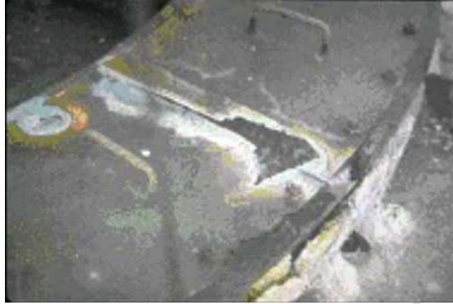
Figure 18—Dew Point Corrosion from Flue Gas Corrosion on Radiant Section Header Box
