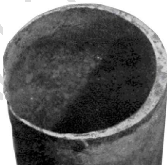
Figure 9—Inside Diameter (ID) of Fireside Portion of Tube Showing Severe Corrosion
