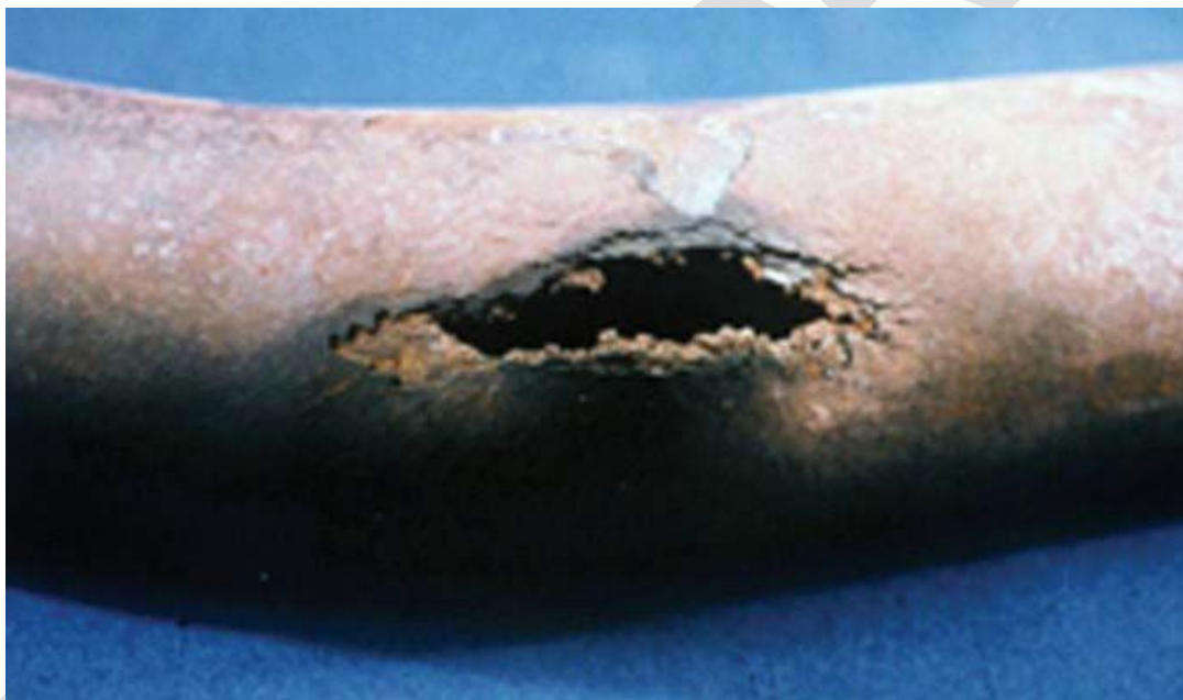
Figure 17—Longer-term Boiler Tube Failure Caused by Poor Circulation and Subsequent Overheating, Oxidation, and Final Failure by Stress Rupture
