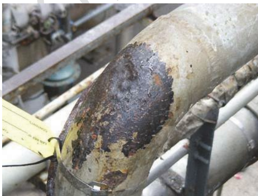
Figure 2—Jacketed Piping with Missing Insulation Plug (top photo) Allowing Water Ingress and
