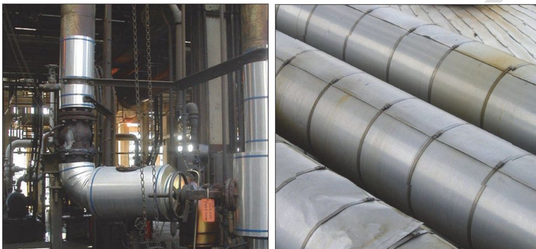
Figure 3546—Examples of Joints with Poor Ability to Shed Water
