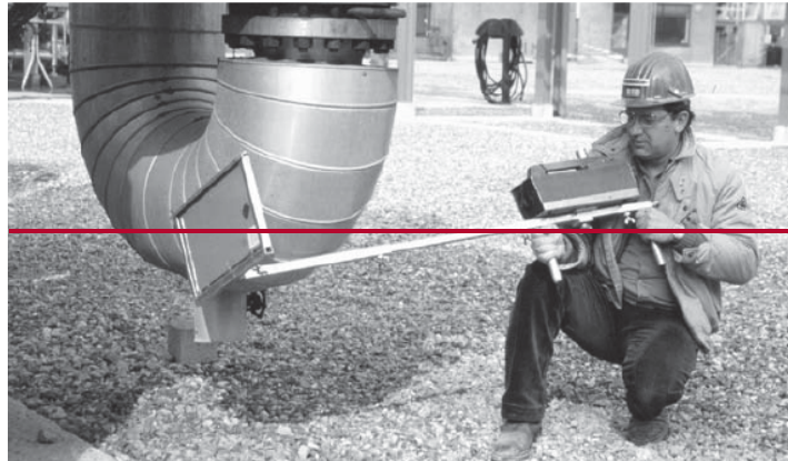
Figure 14—Photo of a Flash Radiography System for Pipe Profiling to Detect Wall Thinning Due to Corrosion
