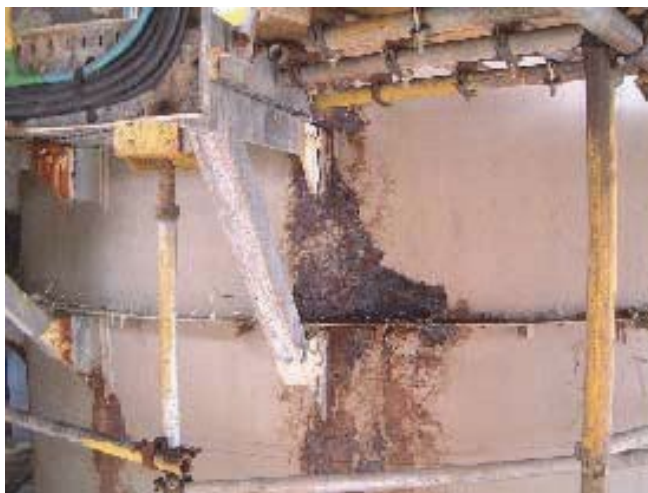
Figure 2635 —Example of a Design/Layout That Is Difficult to Insulate
