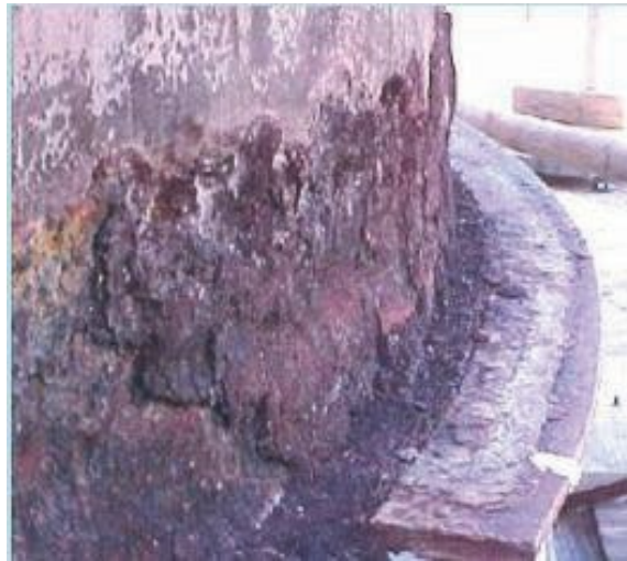
Figure 4—CUI at an Insulation Support Ring
