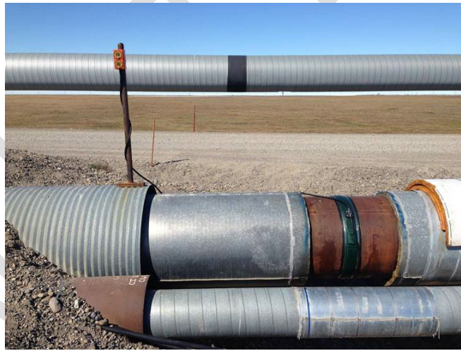
Figure 10: 9—Permanently Installed Monitoring Array of Transducers (courtesy of Guided Ultrasonics Ltd.)
