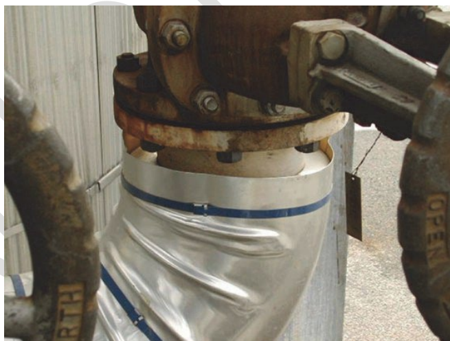
Figure 3647—Example of Missing End Cap
