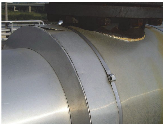
Figure 3344 —Example of Jacketing Joint with Missing Caulking
