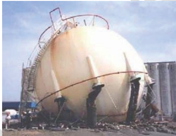
Figure 5—Failure of Sphere Legs Due to CUF
