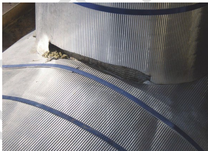
Figure 3445 —Example of Poor Jacketing Fit-up
