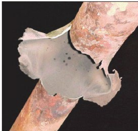
Figure 3—CUI Failure of 4 in. Gas Compressor Recycle Line
