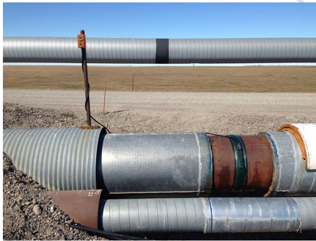
Figure B.7: Permanently Installed Monitoring Array of Transducers
