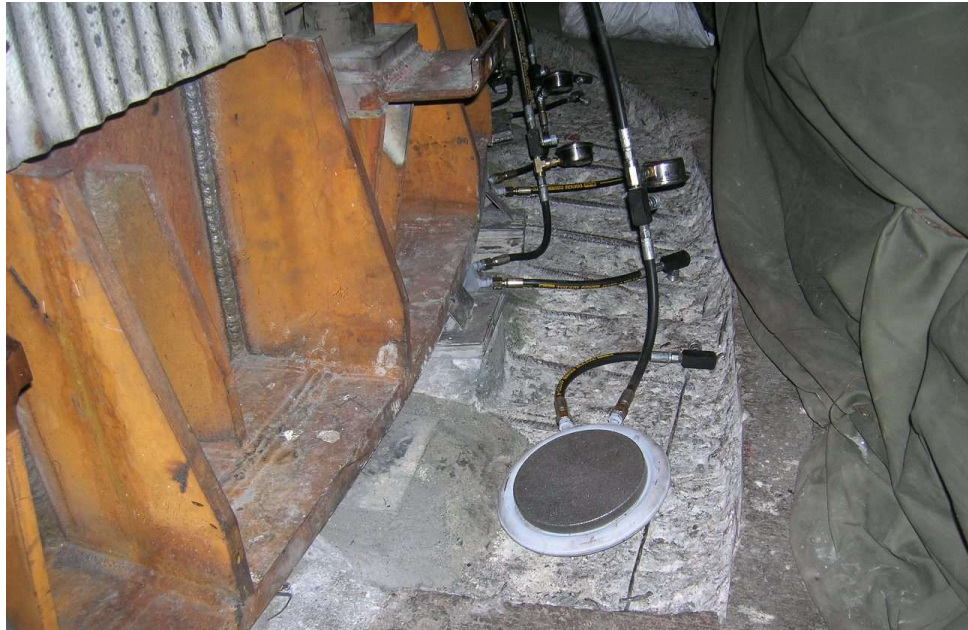
Figure 61—Modifications of Base Ring, Including New Gusset Plates and Positioning and Installation of Multiple Flat Jacks
