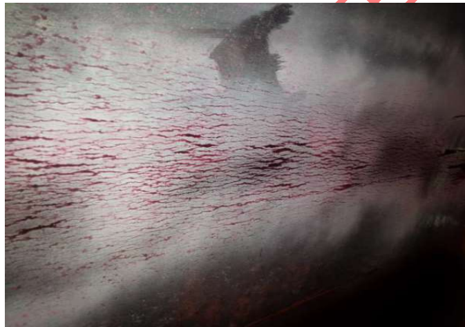
Figure 13—PT from the Outside Surface Displays an Area with “Elephant Skin” Cracking
