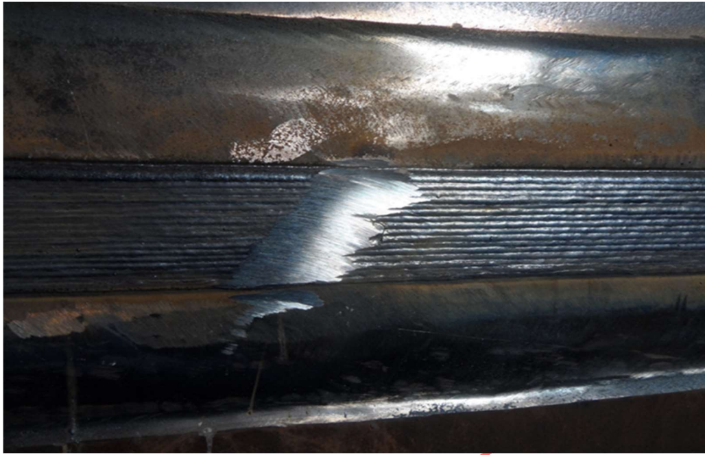
Figure 67—Through-wall Crack Repaired
