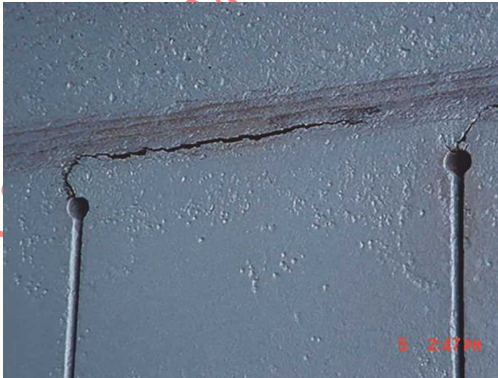
Figure 6 - Keyhole Skirt-to-Bottom Head Weld Cracks
