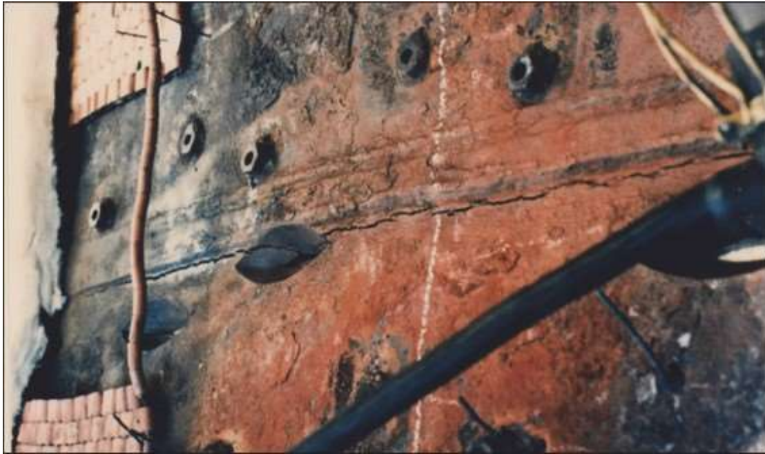
Figure 5 - Typical Cracking Observed at Skirt-to-Bottom Head Weld
