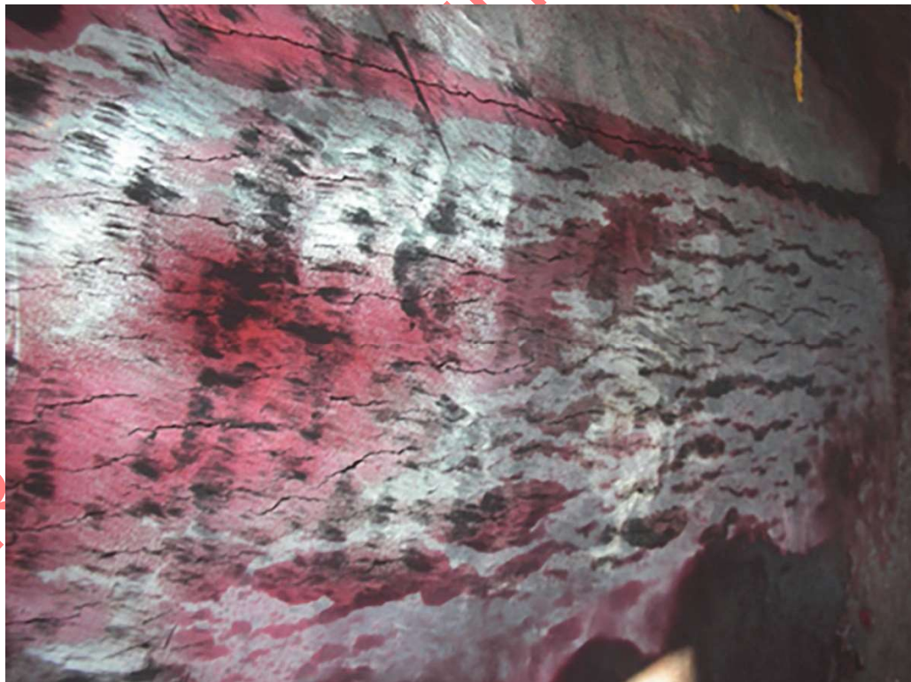
Figure 8b - External Surface Bulge Cracks
