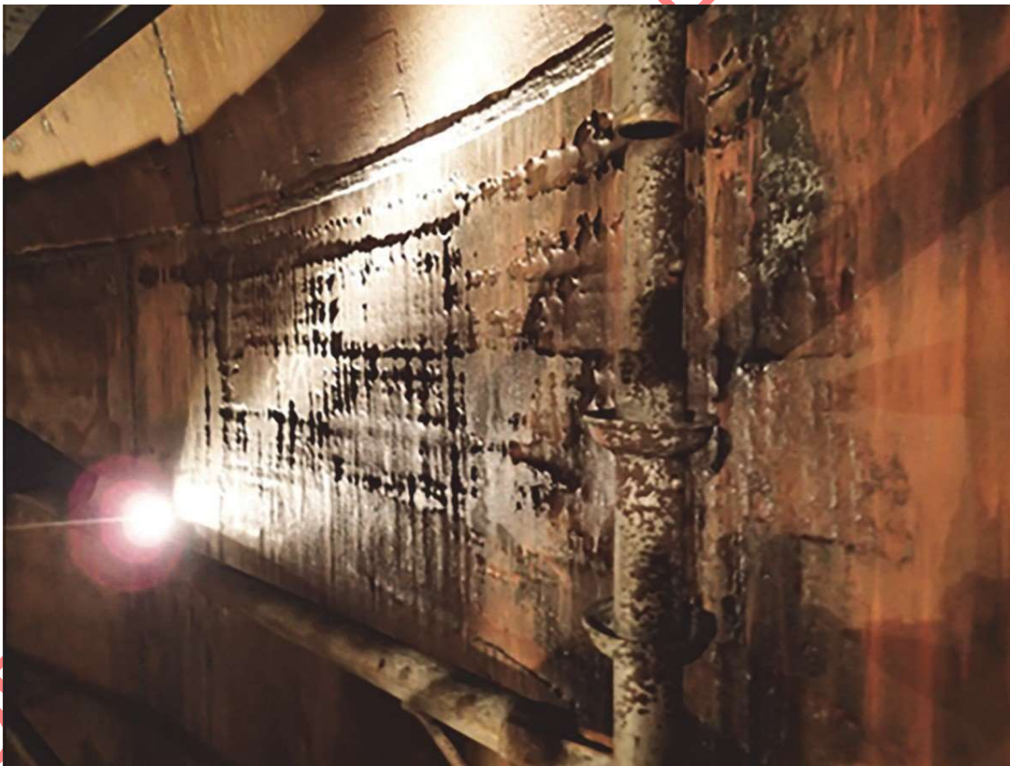
Figure 10 - Corrosion of 12Cr Stainless Cladding in a Coke Drum Upper Section
