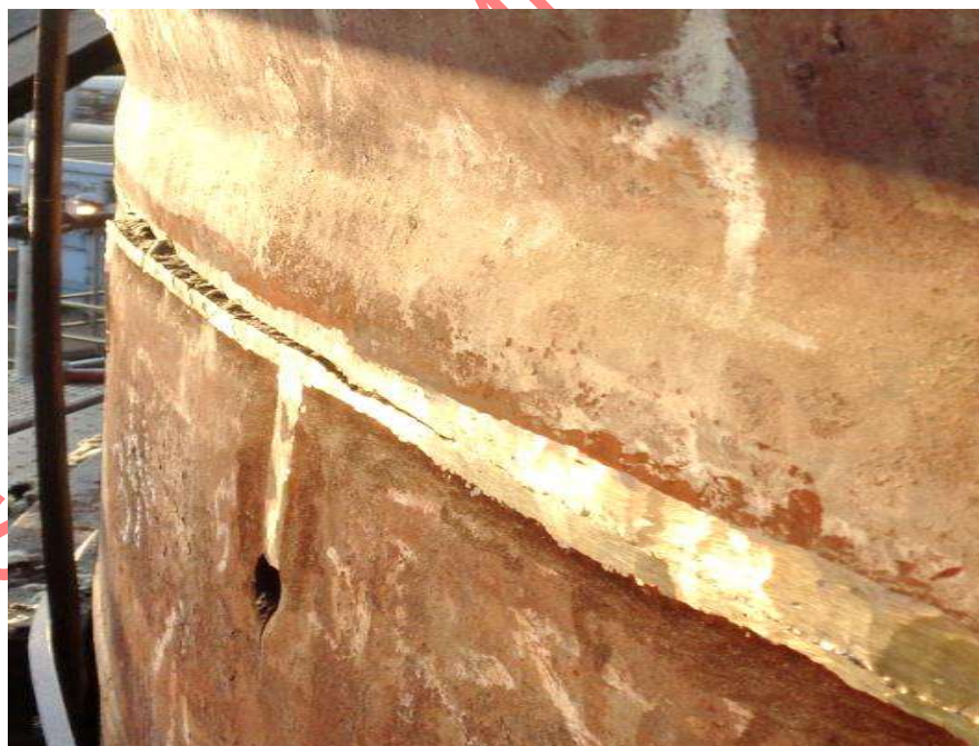
Figure 50—Cracking Initiated at the Slot Keyhole and Propagated Through the Skirt Attachment Weld
