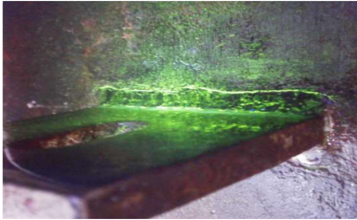
Figure 14—Cracking On the External Surface at an Insulation Clip Displayed by Wet Fluorescent MT
