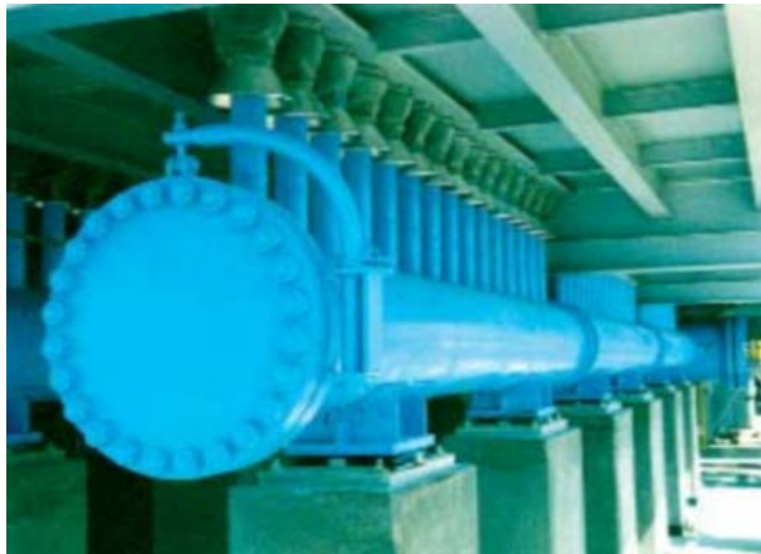
Figure D.4 – Cold Wall Process Gas Outlet Header
